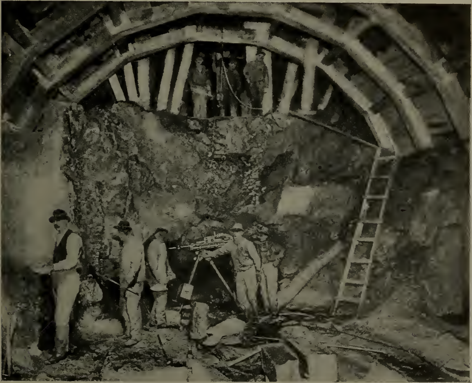
Subway Tunnel Heading at 116th Street and Broadway: Timbering in Soft Ground Over Rock.
